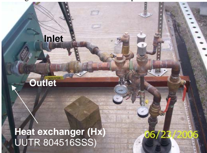
Figure 2A Heat Exchanger Section (On top of container)
