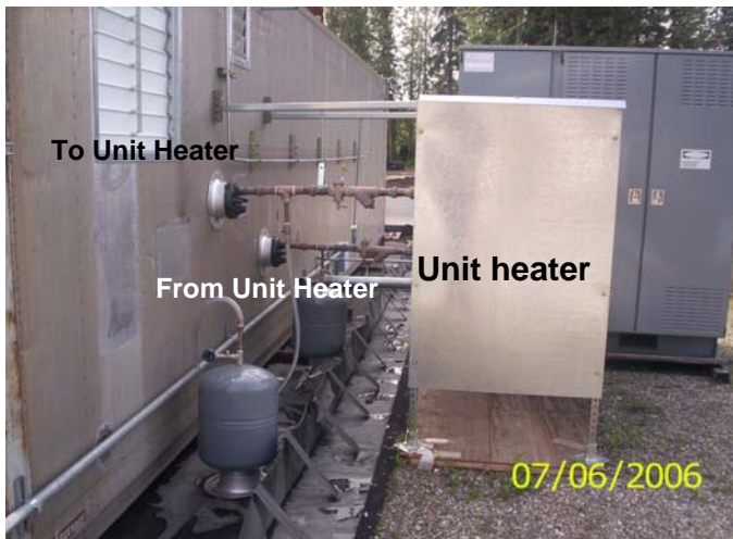
Figure 2B Unit Heater Section (Outside of west sidewall of ISO Container)
